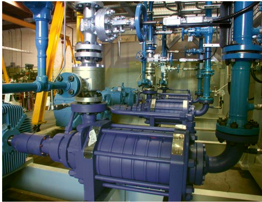
Fig. 3: Twenty SSV valves incorporated protect the pumps in the Oil Sands projects
